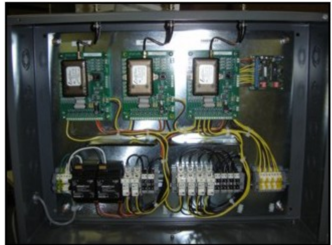
Modified RCD- 6 EAS System with 3 Receivers for Redundancy. Setup for Printer, LED Sign and Audio.
